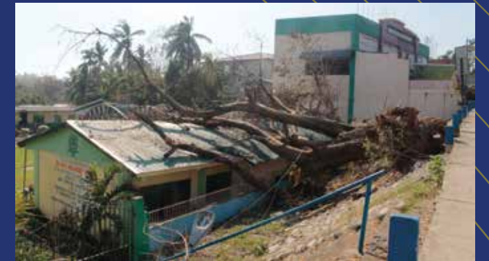
Typhoon Haima damage
